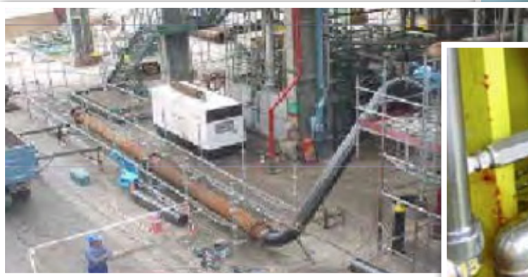
PIPES SET UP FOR LOW AND HIGH PRESSURE HYDRAULIC SYSTEMS
